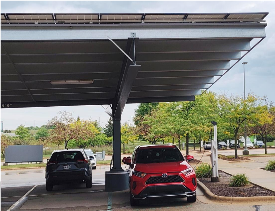
EV car charger with connected solar panels at the Alliant headquarters
